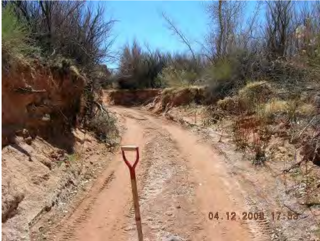
Erosion on Horse Canyon road on steep sections
